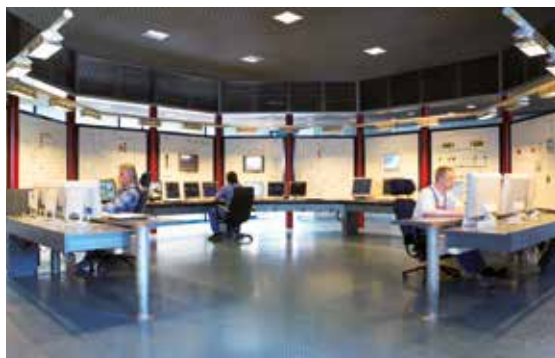
The modern control centre has an overview of all the different data and values. These are continuously being evaluated and automatically fed straight away into the control system. The emission data is forwarded online to the Environmental Protection Agency
