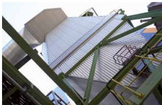
Each of the GMVA's four incineration units has its own separate flue gas cleaning system
